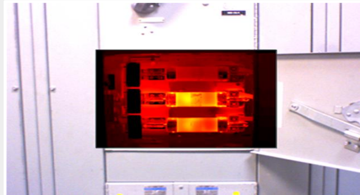
Motor control center
